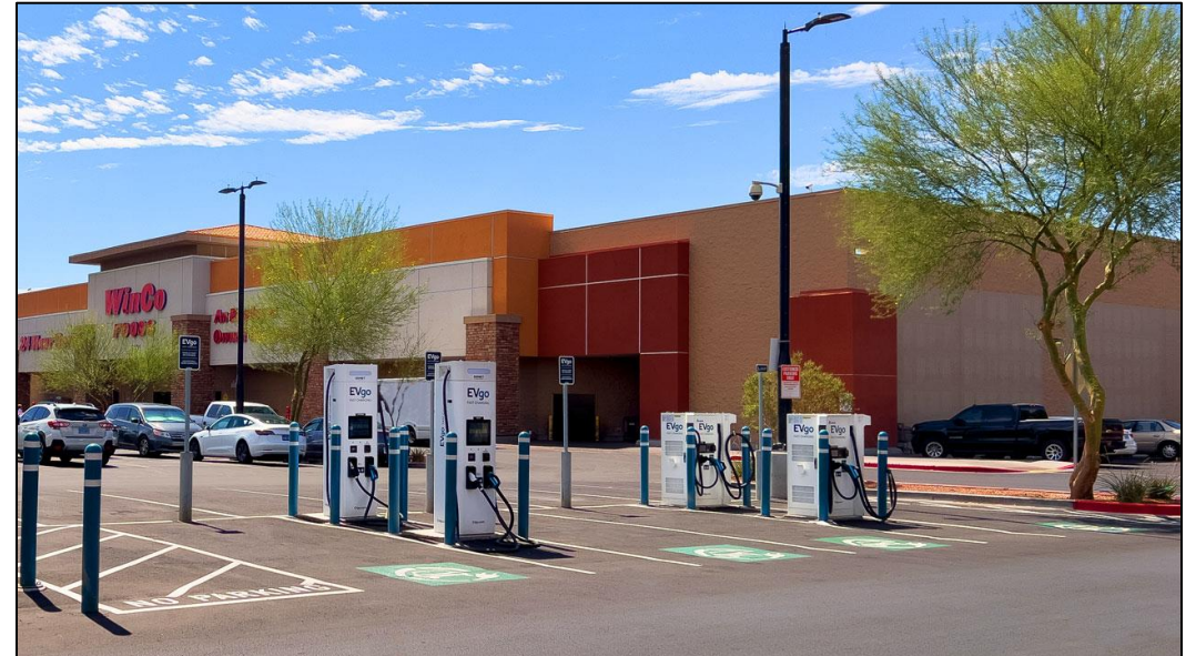
New EVgo chargers at WinCo Foods in North Las Vegas
